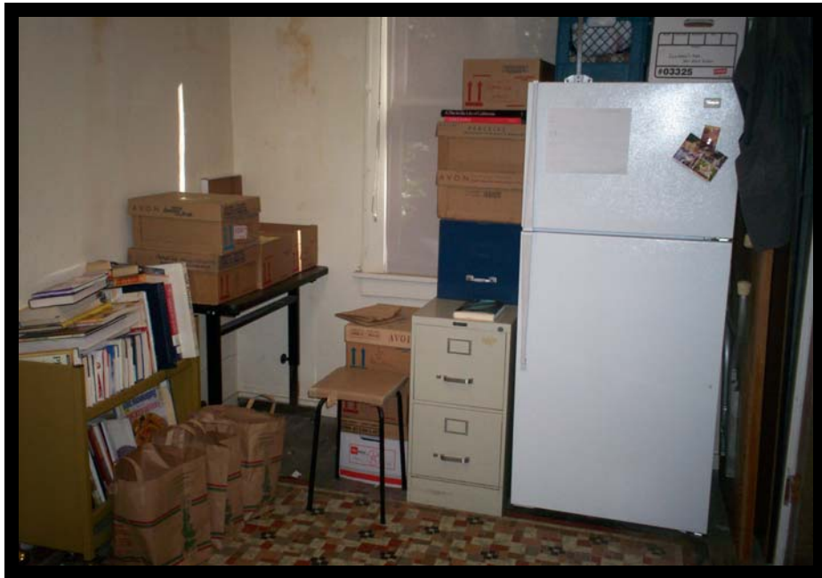
Cluttered Staff Area
