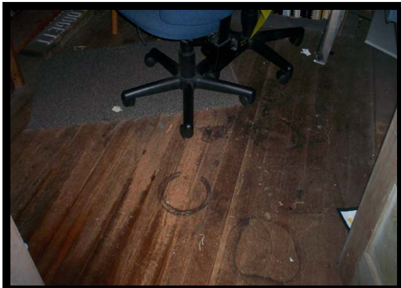
Worn out floors.
